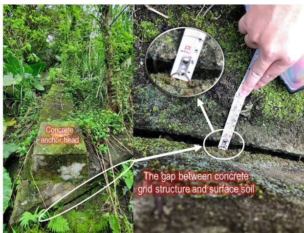
Fig. 12 Gaps between the concrete grid beam and the ground surface observed from the anchored slope (1–2 cm)
